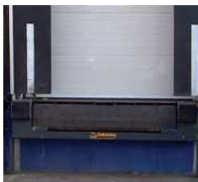
Minidock on a loading bay.
