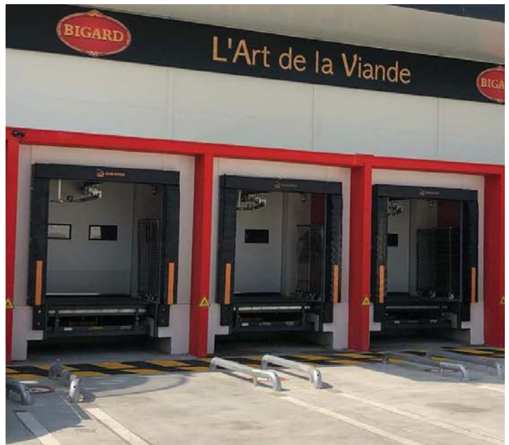
Refrigerated dock shelters are installed directly on the façade.
