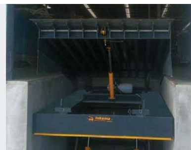
Dual SR Lift Table installed as a loading bay.
