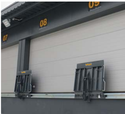
They are perfect for installing as a loading dock.
